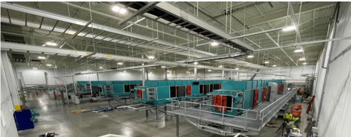
Additional machinery being installed through Q3 2024
